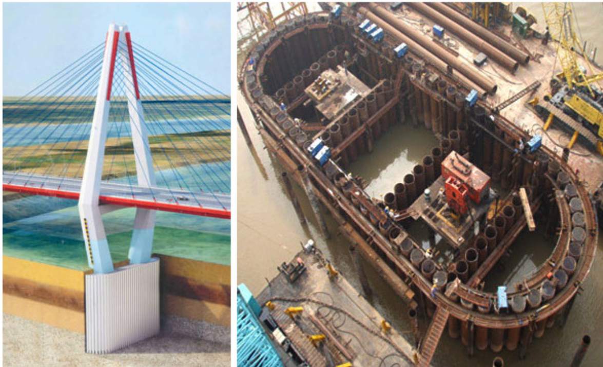
Aerial view of completed installation of steel pipe sheet pile for cofferdam
