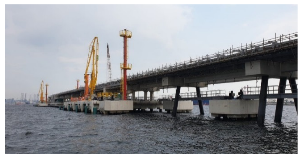
1,000 DWT/20,000 DWT Berth. Both berths connected to Main Trestle by an Elevated Trestle
